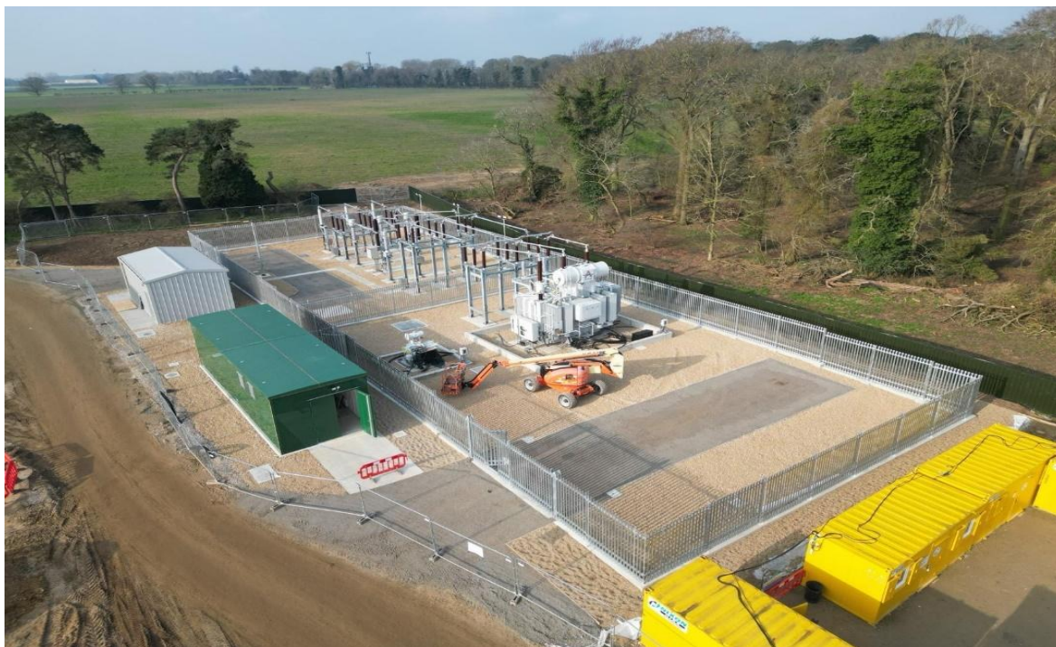
Image 4.8: 132/33kV Substation (Single Transformer)
