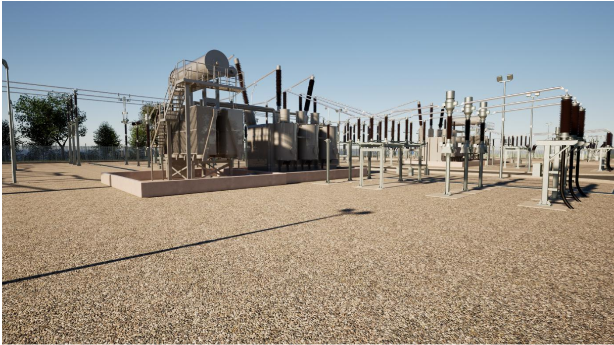
Image 4.9: Typical 400kV Power Transformer
