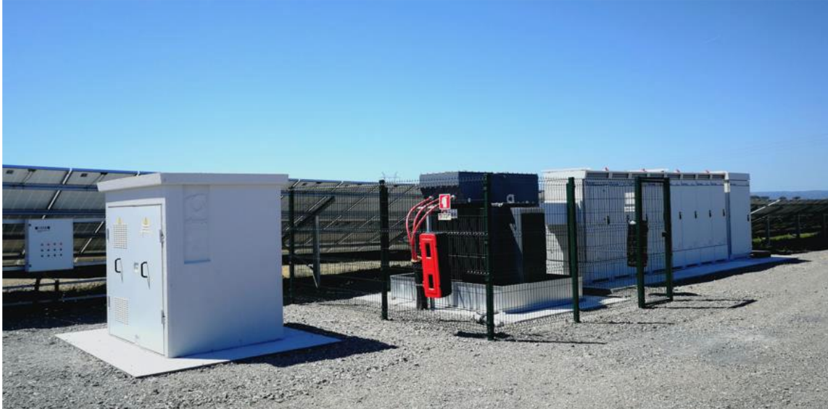
Image 4.4: Typical Standalone Conversion Unit
