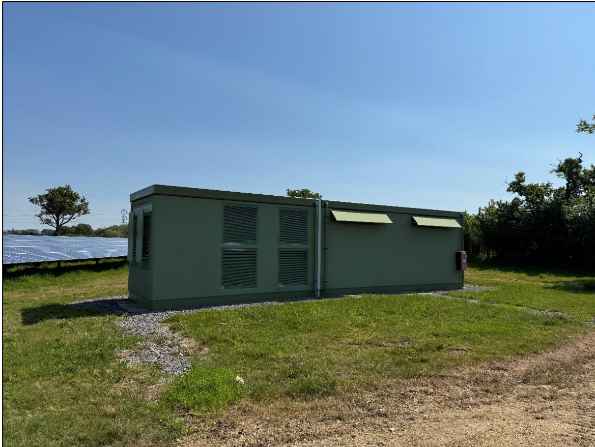
Image 4.6: Typical Conversion Unit / 33kV Sub-distribution Switch Room
