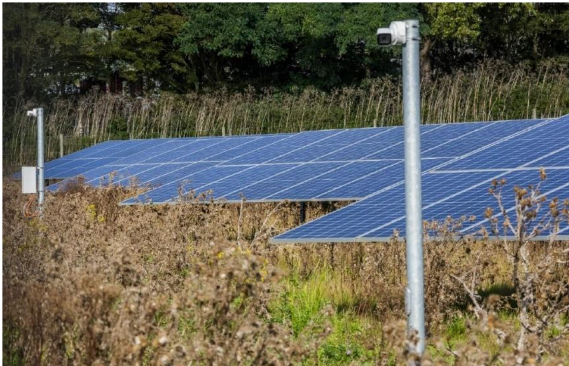
Image 4.15: Pole-mounted Security Camera (unpainted)
